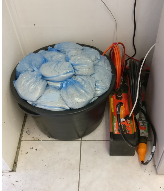
Figure 9. Seismic installation at station SABV. The seismometer rests on the tiles on the concrete floor and is completely surrounded by dry sand in a quasi-flexible container. Next to the sensor is the datalogger.
