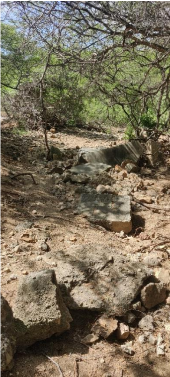
3=big maintenance should be done
