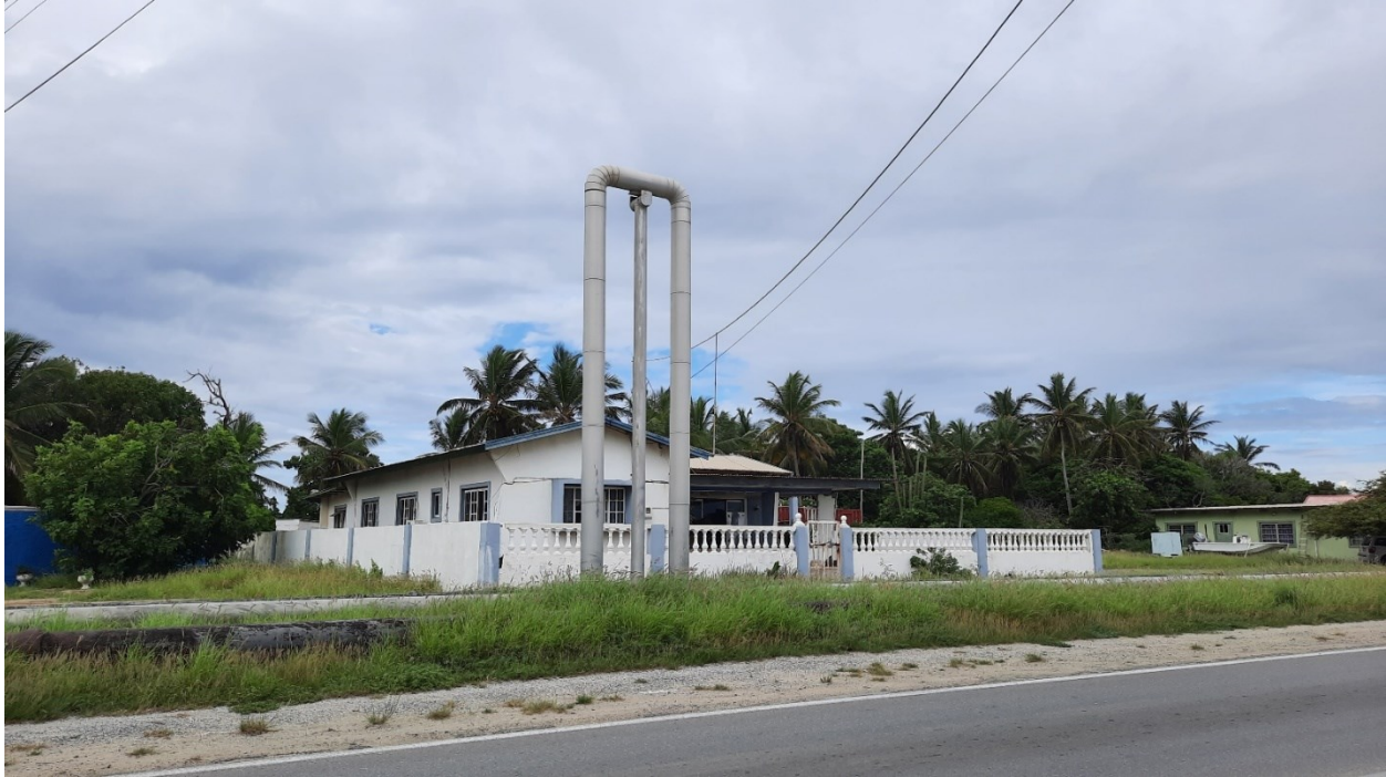
Figure 3: Proximity of existing pipelines to houses (Diario, 2022c)
